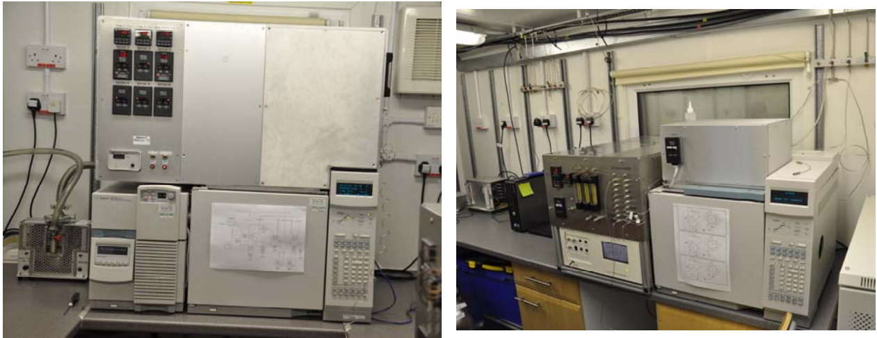
Figure 4: The Medusa (left) and MD (right), installed and running samples in the Mobile Lab.
